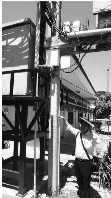
Dr. Komchit Chavanasporn, member of HOPE Assessment team, inspects the elevated electrical circuit board which was raised to a higher level after flooding which hit Ayutthaya Hospital
