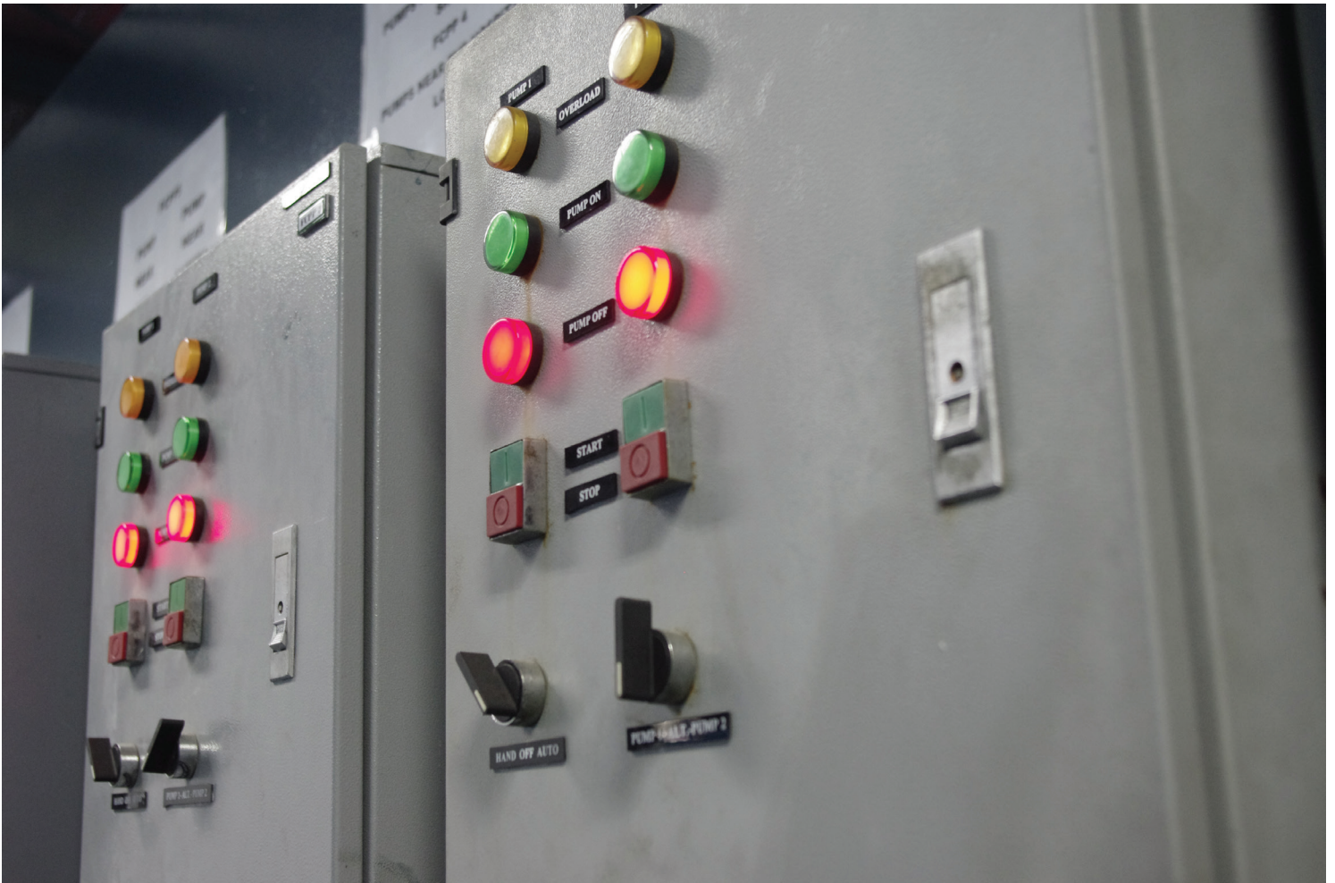
The pumping machines at UERM Medical Center automatically start pumping floodwater back in the river when the water level reaches a certain height. The modern monitoring boards make it easy to oversee the pumps that are tested every month.
