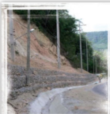
Gabions, cages filled with rocks, sand or soil, help to stabilize the slope from erosion. Image credit: RECLAIM
