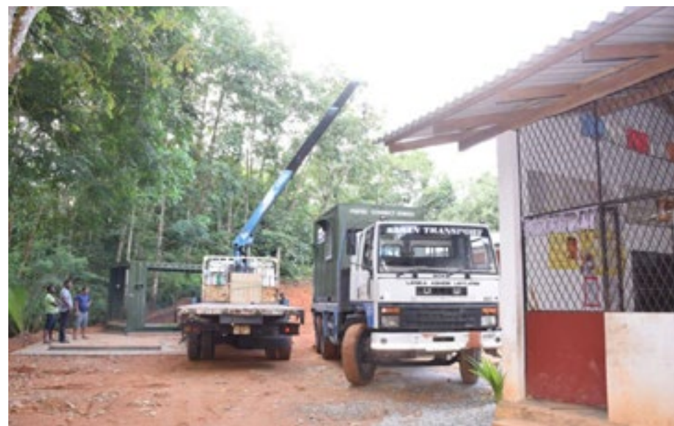
Installation of model camp management site at Kithulegoda primary school. Photo by Janathakshan GTE Ltd.
