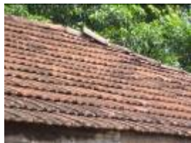
Damaged roof due to wind
