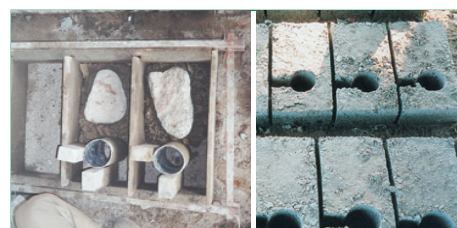
Broken stones from demolished school buildings are filled into molds (left) to make stonecrete blocks (right)
