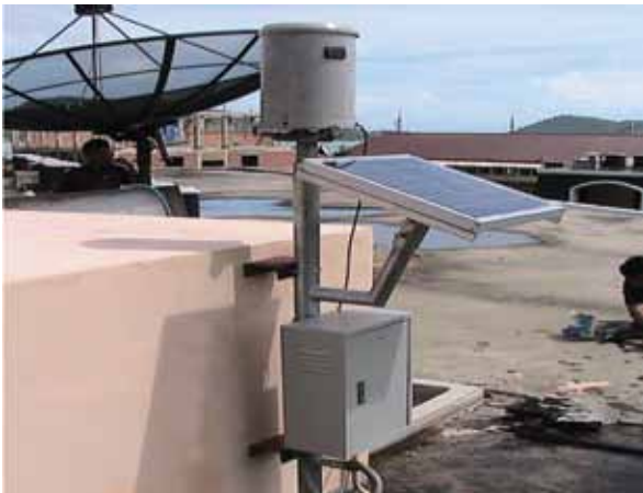
Automatic wireless rain gauge system with GPRS, Patong City, Phuket, Thailand
