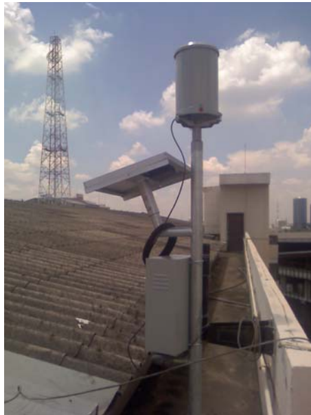
Figure 6-22 Automatic wireless rain gauge system with GPRS
