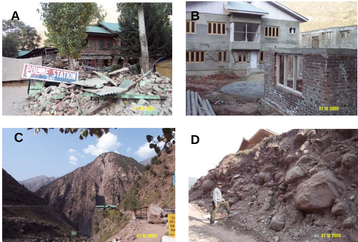
Figure. 8a). Complete collapse of Police station at URI town ( 34^{\circ} 04' 36.0'' , 74^{\circ} 03' 56.8'' ), b). The earthquake surveyed partially constructed house and at the back ground the large diagonal cracks in the side walls of the house, but the walls have not failed, c). The fresh landslide in the steeply dipping hard red color sandstone of Murree Formation, at red bridge ( 34^{\circ} 06' 03.3'' , 73^{\circ} 57' 29.1'' ), d). Fresh land slide in the thick colluvial deposit near Urusu village along the National High way leading to Muzafarabd ( 34^{\circ} 06' 25.9'' , 73^{\circ} 56' 00.4'' ).
