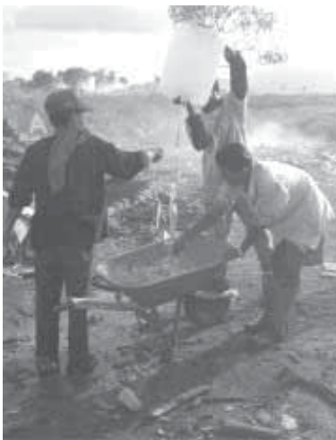
About 500 Acehnese have been hired by a UNDP recycling programme that is turning tsunami debris into reusable materials
