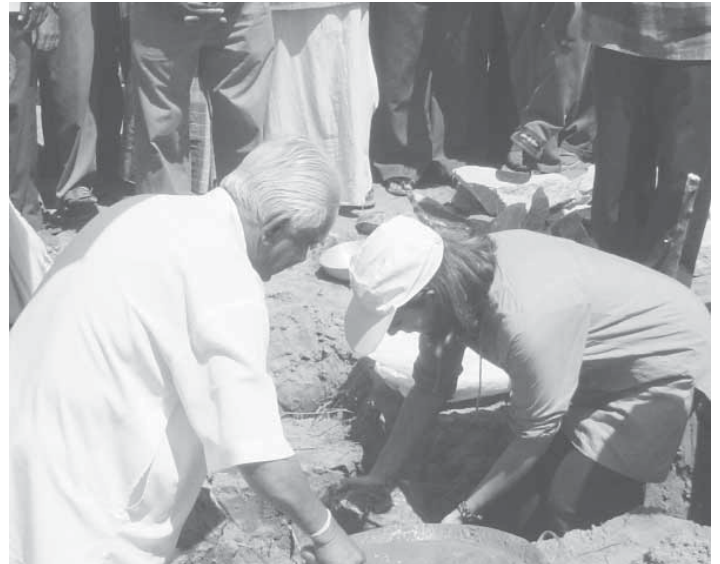
Dr A T Ariyaratne laying the foundation stone for the Tsunami Housing Project in Vaddavan, a small Tamil village on the east coast of Sri Lanka.
