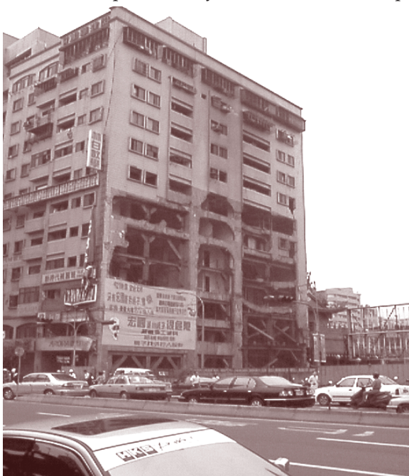
Fig. 1: Building affected by an earthquake
