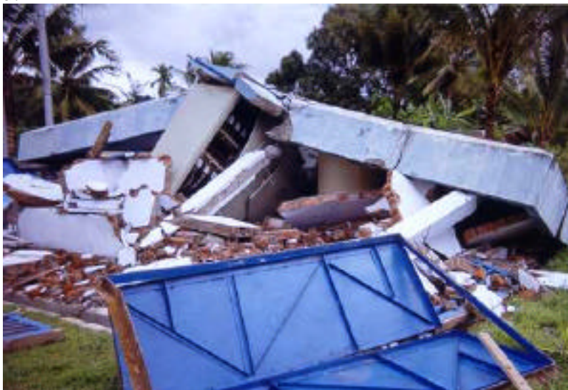
Figure 5 Damaged powerhouse in water treatment plant in Bengkulu City
