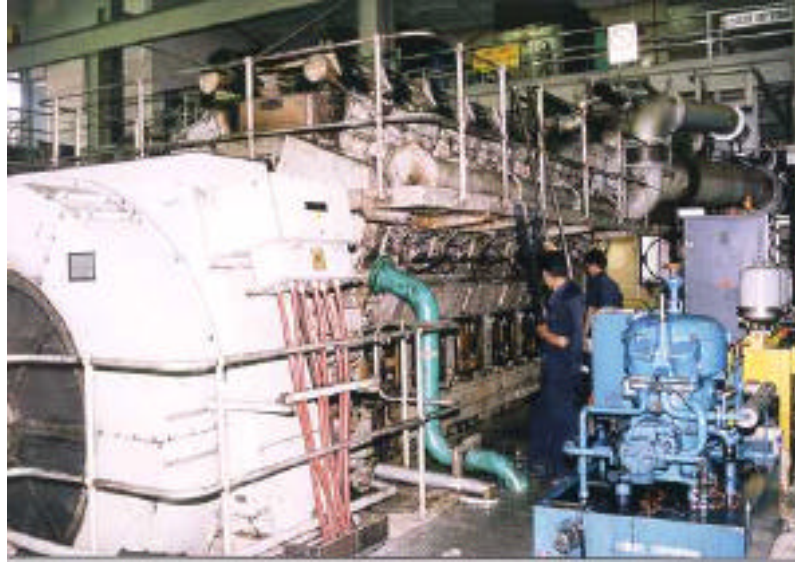
Figure 4 The generator No. 2 at PLTD Suko Merindu is under repair after the earthquake
