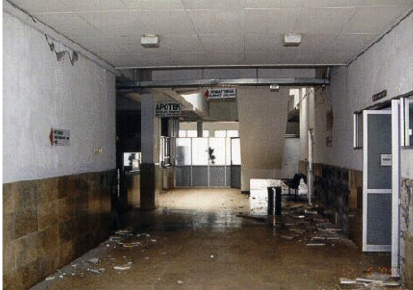
Figure 8 Damaged general hospital in Bengkulu City
