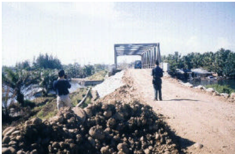
Figure 3 Bridge near the Pulau Baai harbor after temporary rehabilitation
