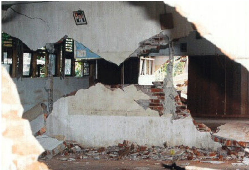
Figure 7 Damaged school in Bengkulu City
