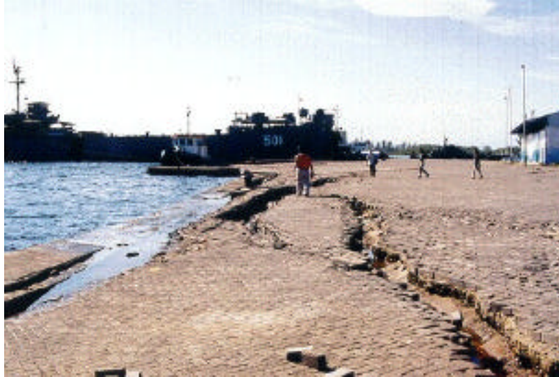
Figure 2 Damage at Pulau Baai harbor
